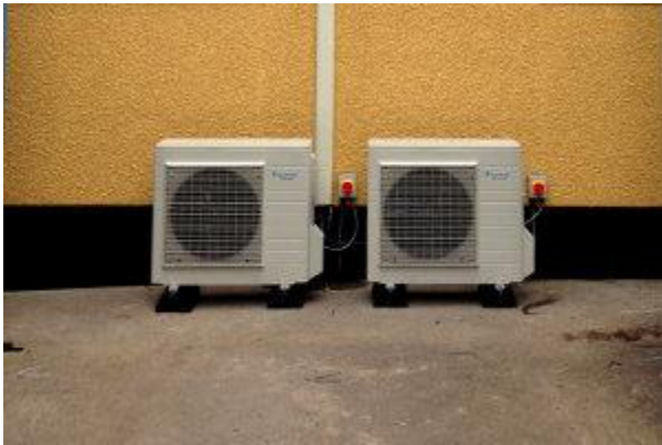
Split System Air Conditioning
